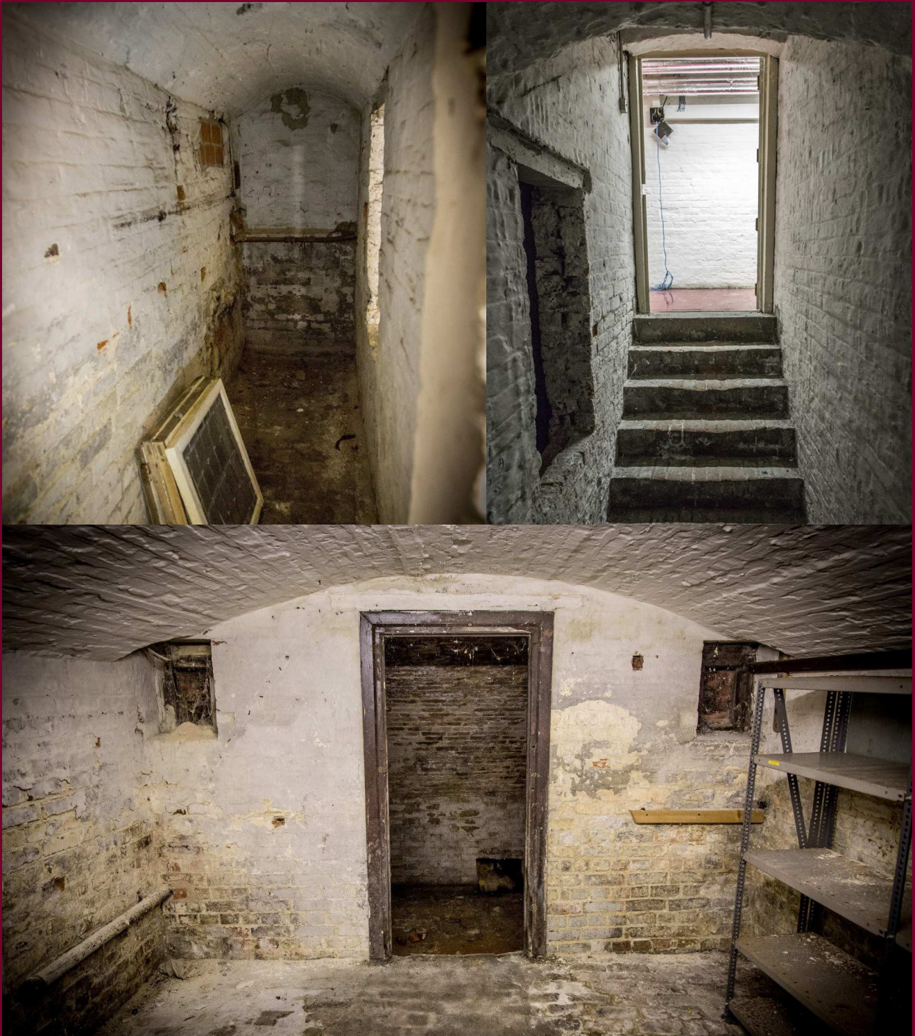
TL - A small corridor off the side of the air raid shelter. TR - The entrance to the air raid shelter from inside the shelter itself. B - The inside of the air raid shelter after the closure of the DPB, although it is likely in a similar, if a bit more dusty, state today.
