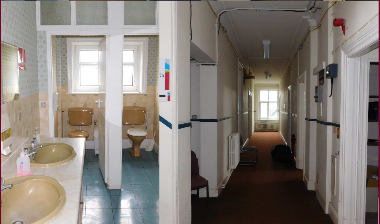
TL - The bridge that links to Block 'D' with the blocking wall just behind the doors. TR - The lift that goes from the 1st floor to the attic, used for heavy goods. BL - The female toilet room that has been abandoned since the DPB's closure. BR - The main corridor on the 2nd floor leading to a fire exit out the side of the building.
