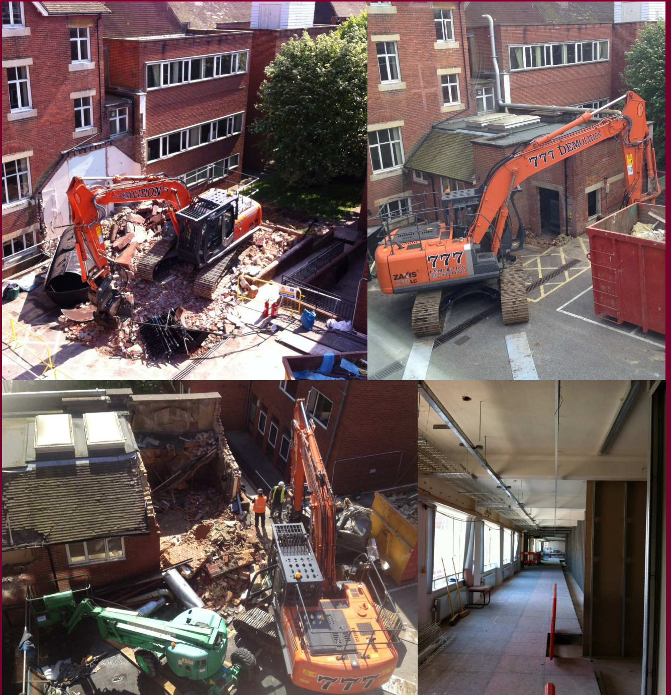
TL - The small building off of Temple Grove after being destroyed. TR - The previously mentioned building before being destroyed. BL - The building midway through its destruction. BR - An unfinished corridor in 2013 that was developed into classrooms.
